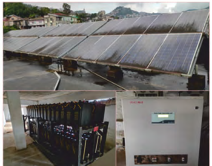
Solar Power System
